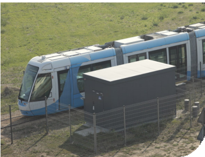
A HESOP substation in testing on a La Rochelle experimental track in September 2009.
